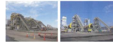
④ Incinerator (Left: Stoker, Right: Rotary Kiln)
